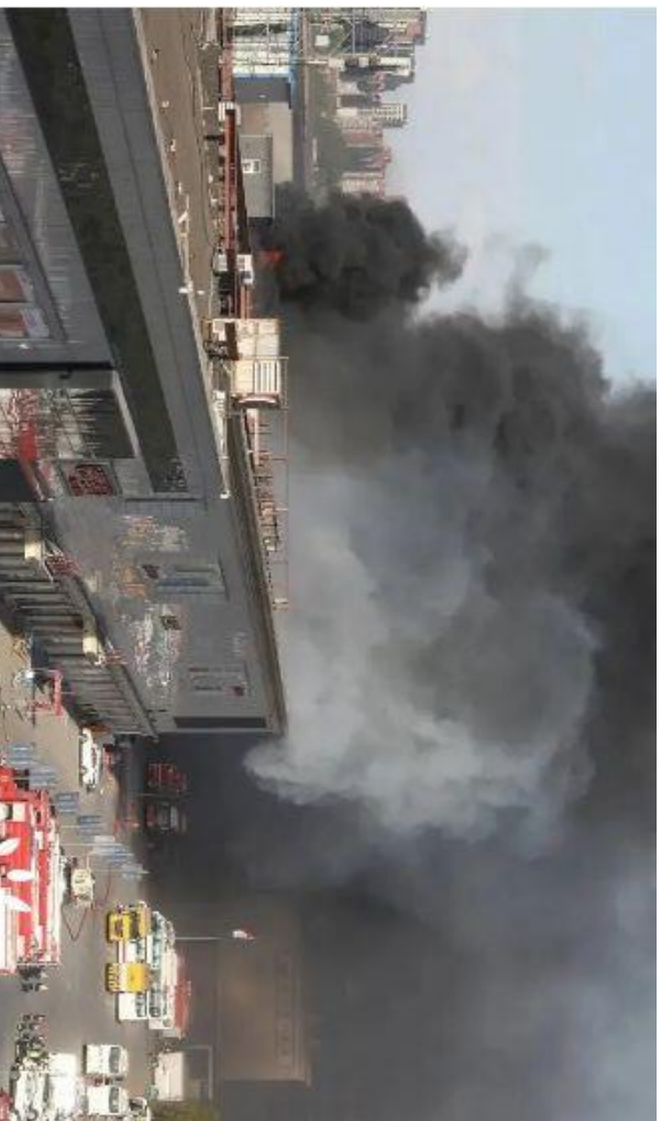
April 16 th , 2021, the 25 MWh energy storage system in Fengtai District, Beijing suddenly exploded. (Battery cell chemistry: LFP )
